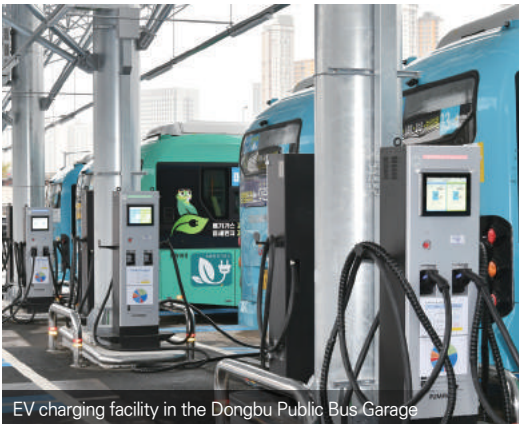
EV charging facility in the Dongbu Public Bus Garage
